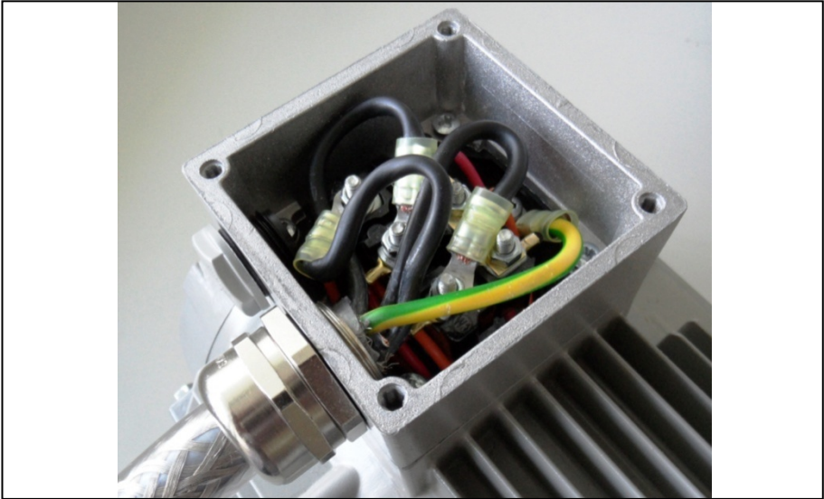
Fig. 26: Wiring on the motor connection box
